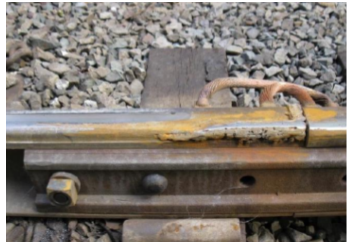
Green Line Rail Damage
