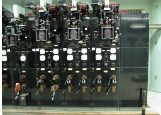
Original Open Faced DC Switchgear
