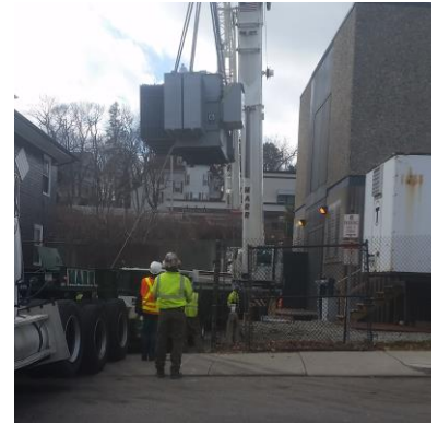
Installation of No.1 RECT TRANS at the at Wollaston Traction Power Substation ACCESS GATE
