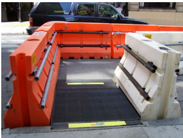
Portable ramp for curb transition into the temporary pedestrian access route
