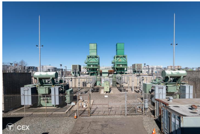
Figure 15: South Boston Power Complex
