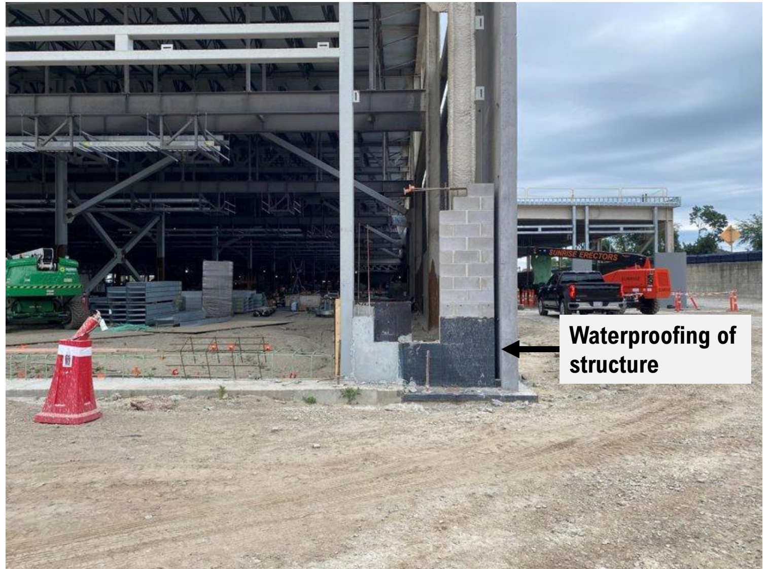
Figure 29: The new Quincy Bus Garage incorporated several resiliency design features, including the building waterproofing shown in the above photo.
