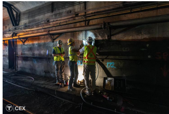
Figure 34: MBTA employees address signal equipment
