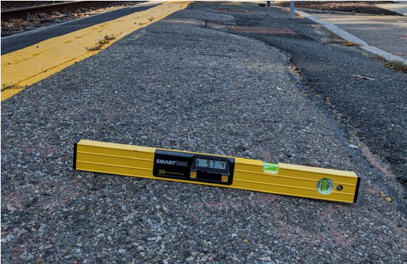
Excessive Cross Slope
