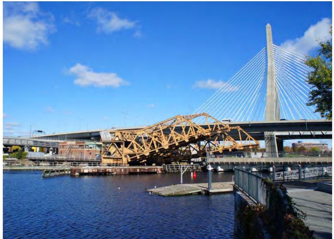
Photo 6 View of existing bridge in partially open position from Nashua Street Park from Boston.
