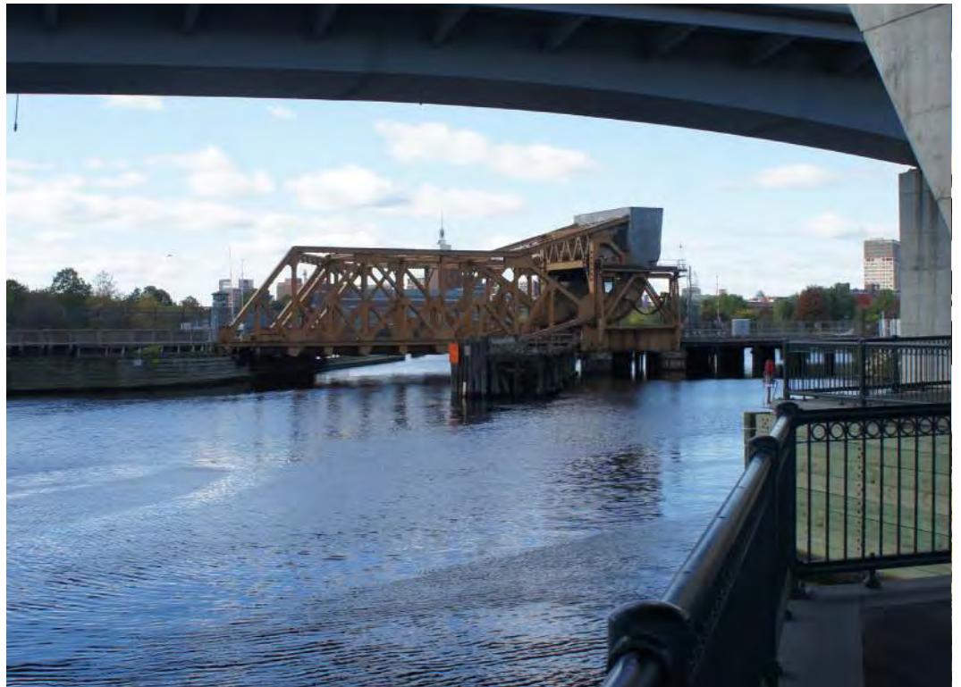
Photo 2 View of Draw One Bridge underneath Zakim Bridge, looking west from Cambridge.
