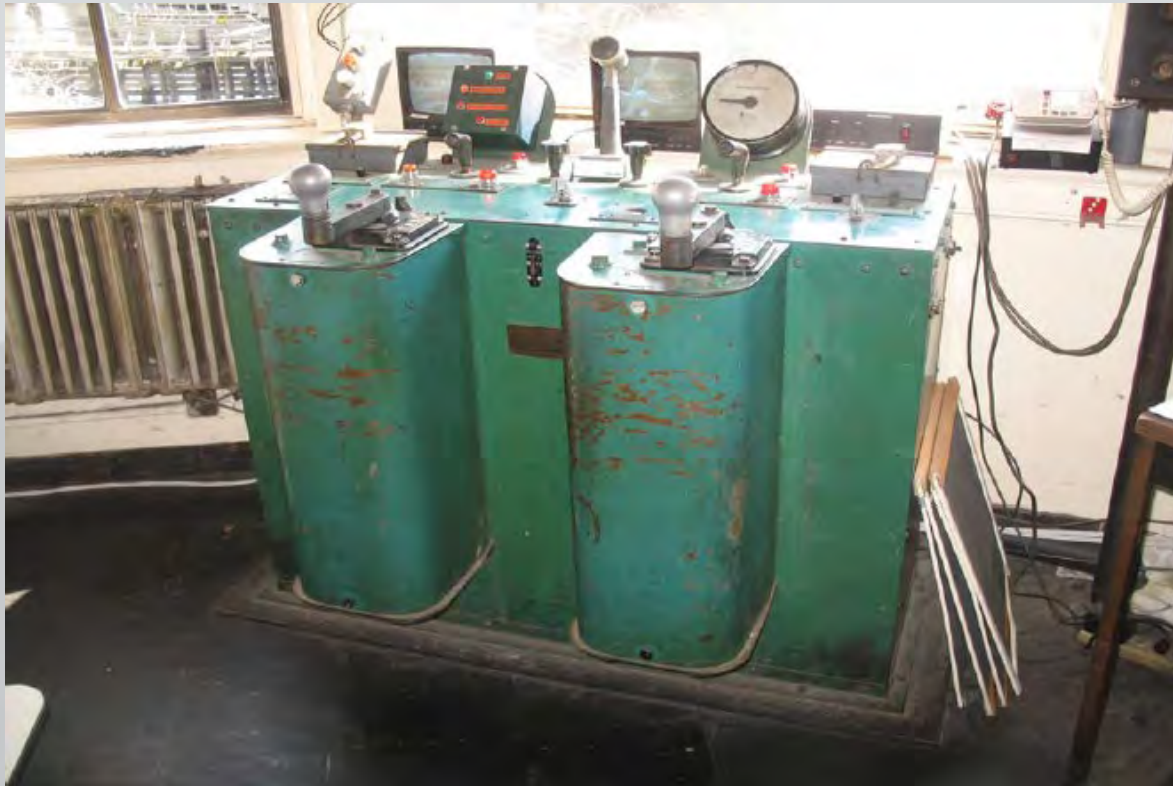
Switching machinery, second floor control room, since moved to current control tower. 2010
