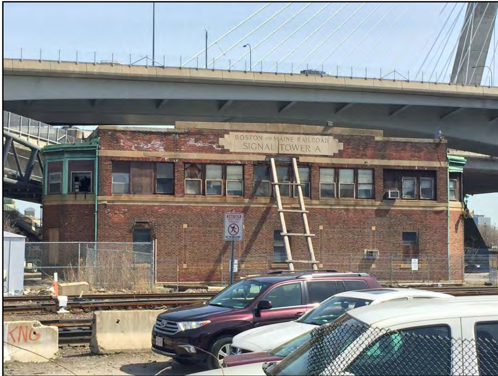
Figure 11. Signal Tower A, looking east at the west (trackside) elevation with temporary timber shoring.
