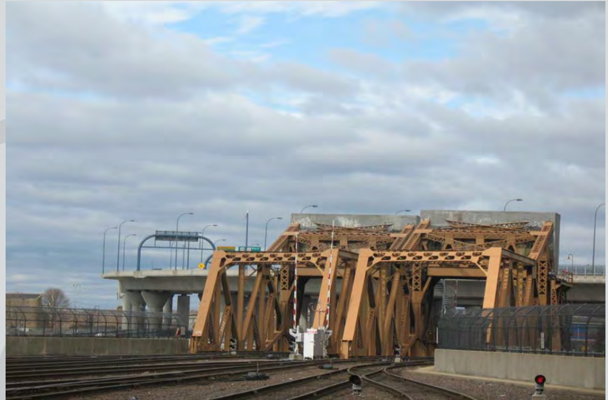
South ends of West Span (l) and East Span (r), looking northwest. 2010
