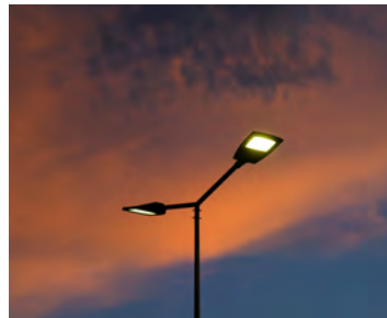
Improving street lighting
