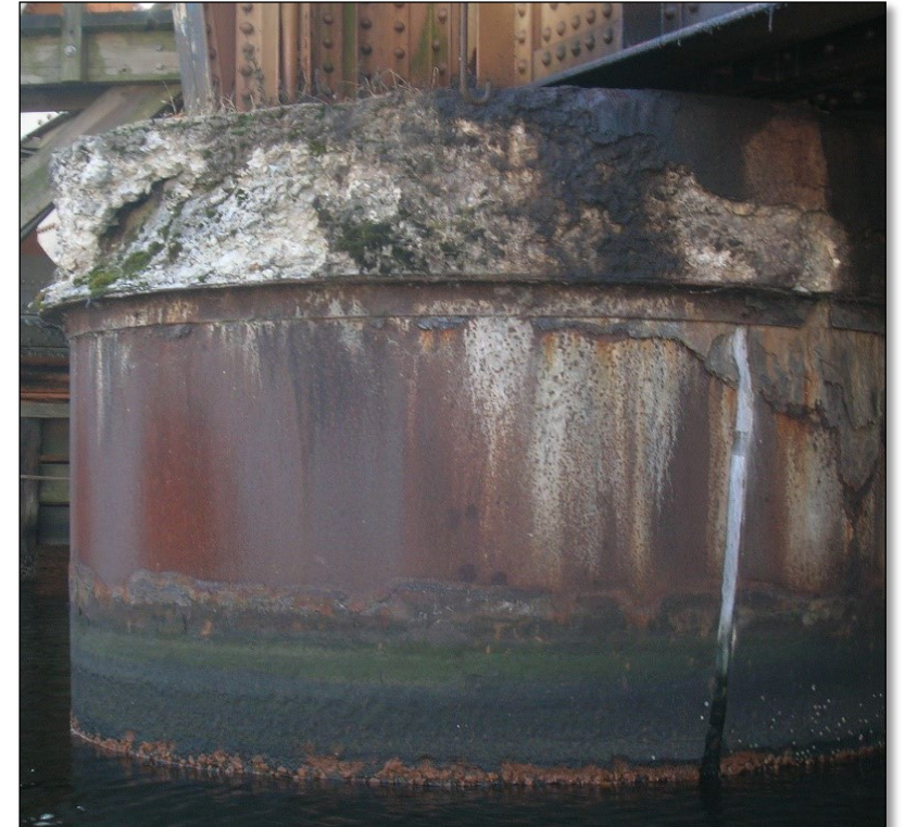
Picture of Bridge Caisson deterioration
