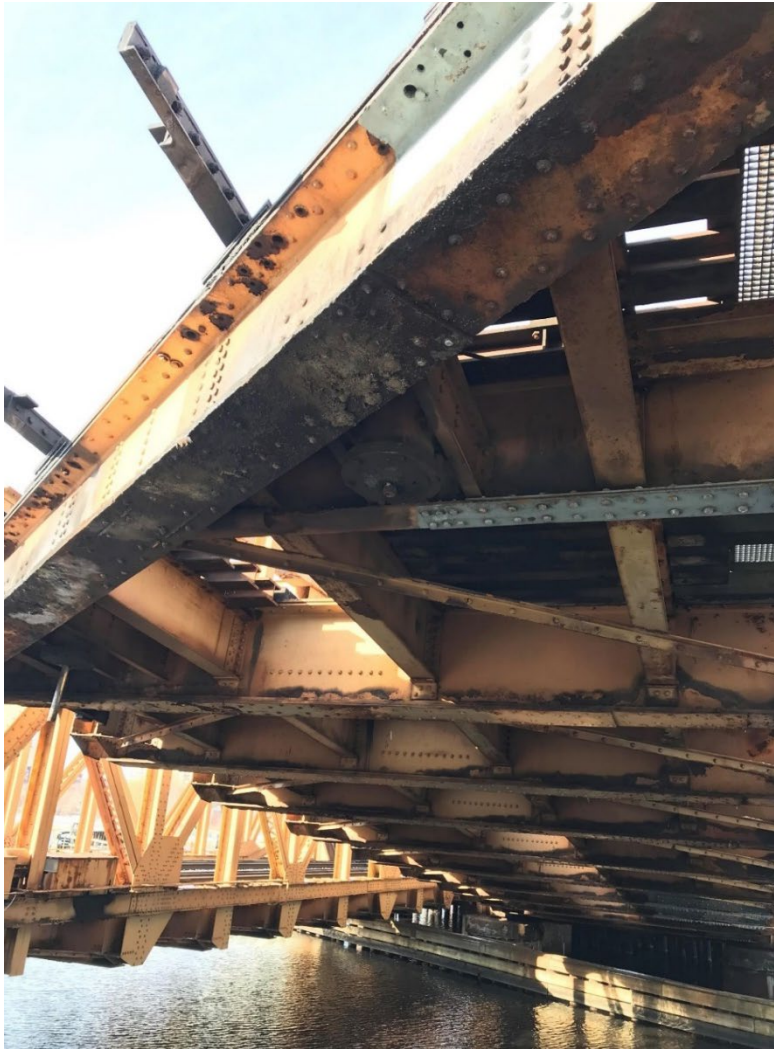
Existing Draw One framing system with deterioration and previous repairs.
