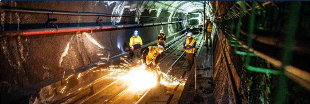
Track work during Red Line diversion as part of the Track Improvement Program.
