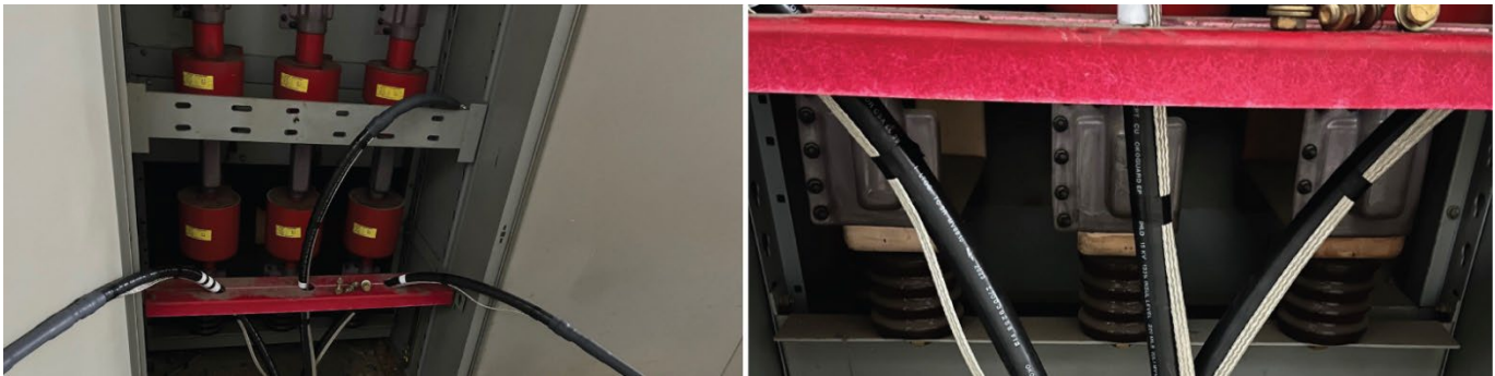
New electrical cables connect Sullivan Station to the traction power substation
