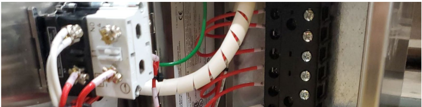
Electrical wiring in Wellington Vehicle Maintenance Facility
