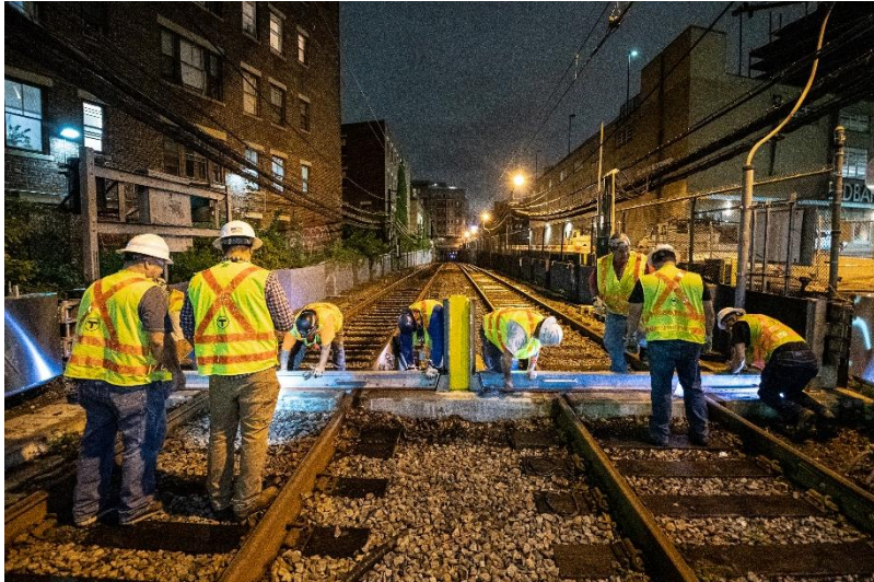
Installation of flood gates on the Green Line's Fenway Portal near Fenway Station
