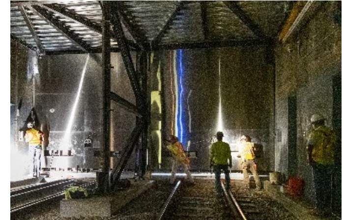
Installation of flood gates on the Green Line's Fenway Portal near Fenway Station
