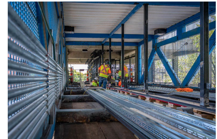
Construction of an accessible pedestrian bridge at the Suffolk Downs Station on the Blue Line
