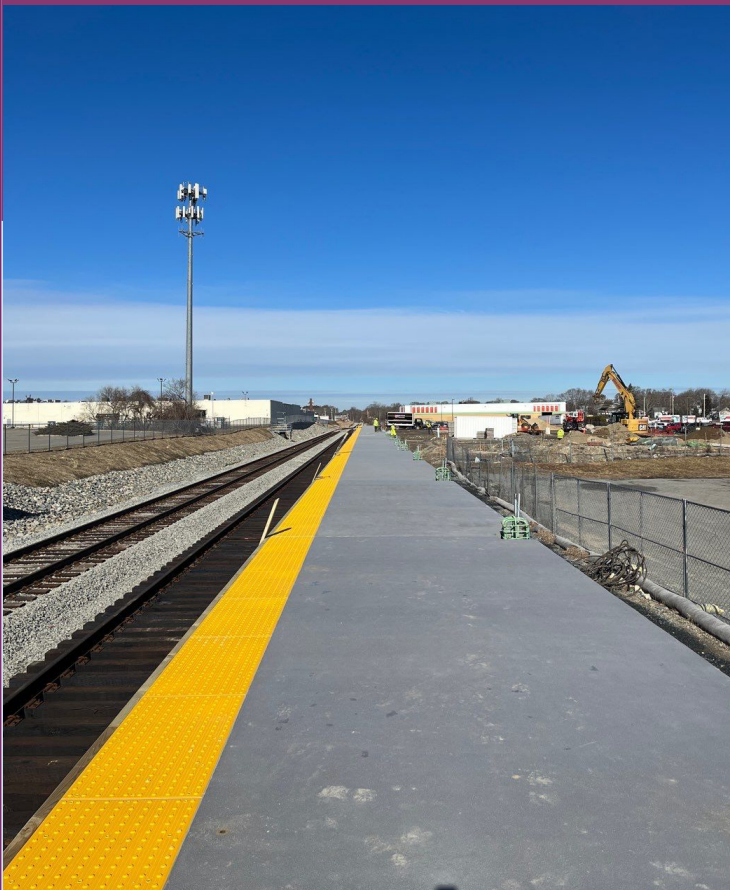
FRP Platforms at Church Street Station in New Bedford, February 2023.
