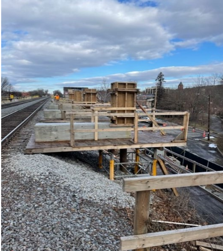
Form work for Platform Light Post Pedestals at the Platform Support Caps on the Outbound Side (February 2023)
