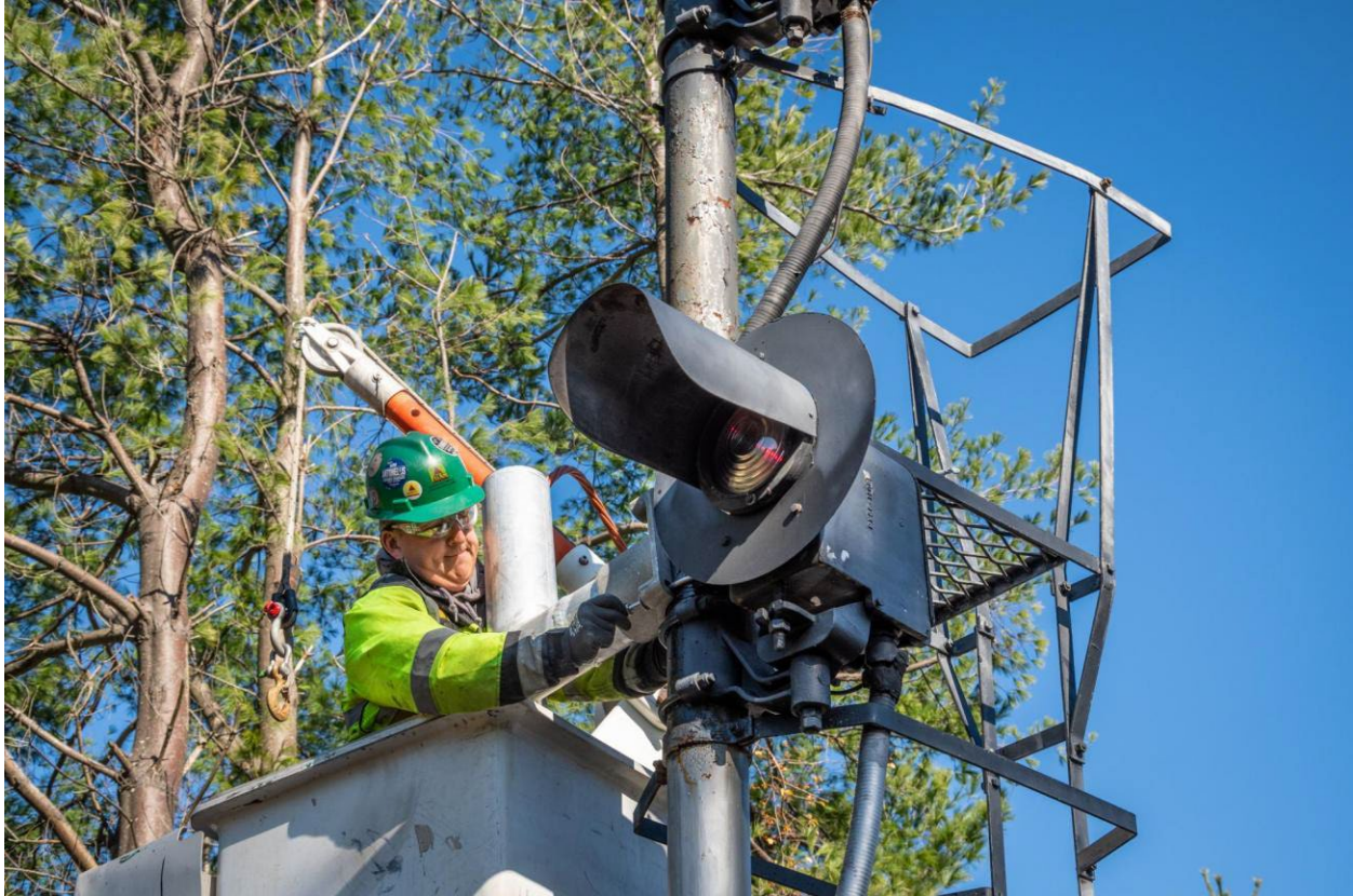
Automatic Train Control
