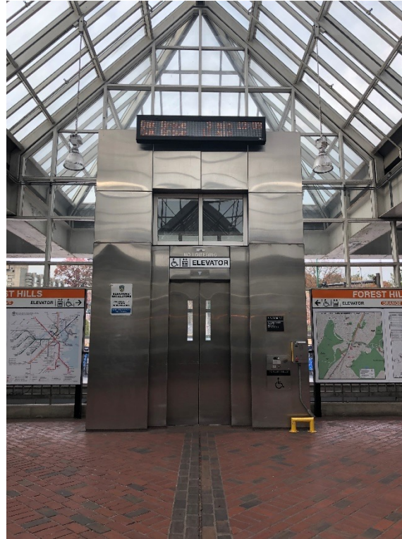
Existing elevators need replacement
