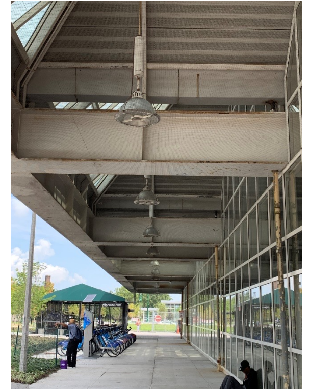
Exterior of building worn down due to decades of exposure
