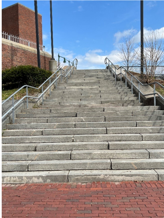
Uneven steps creates potential tripping hazards
