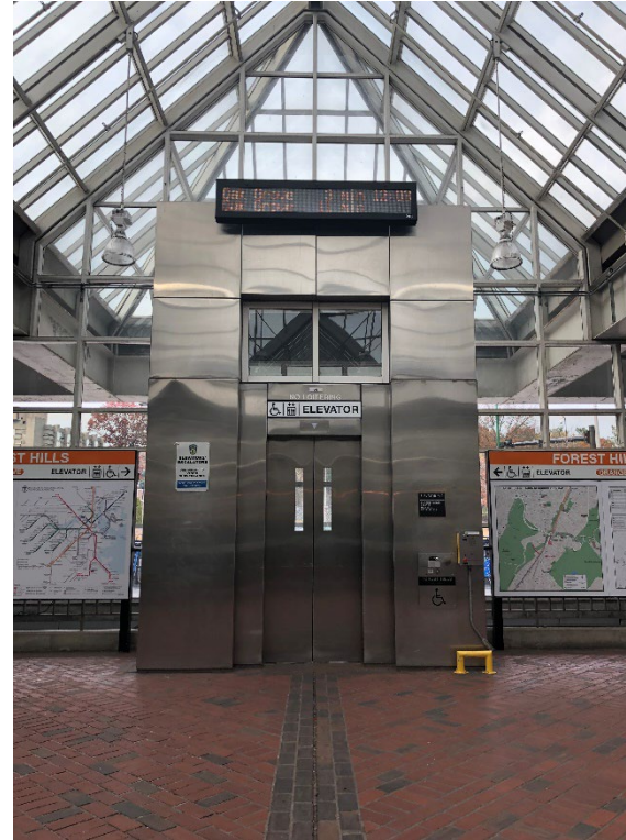
Existing elevators need replacement
