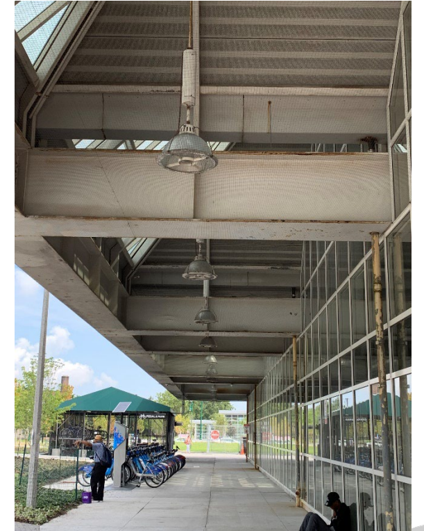
Exterior of building worn down due to decades of exposure
