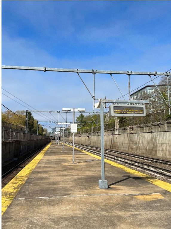
Existing platform requires ADA upgrades
