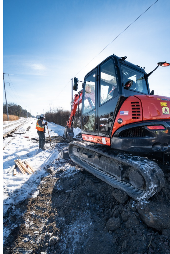
Lowell Line Cable
