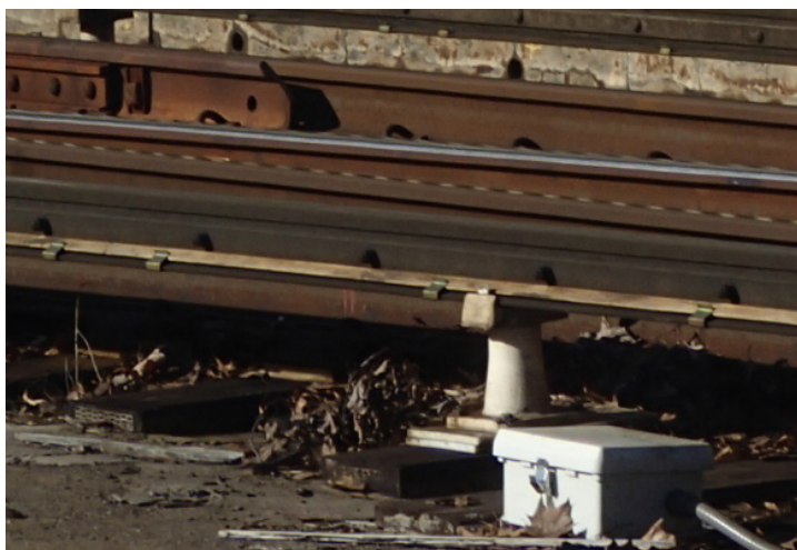
Figure 6.6.3-9 Track Asset Deficiency: Cable
