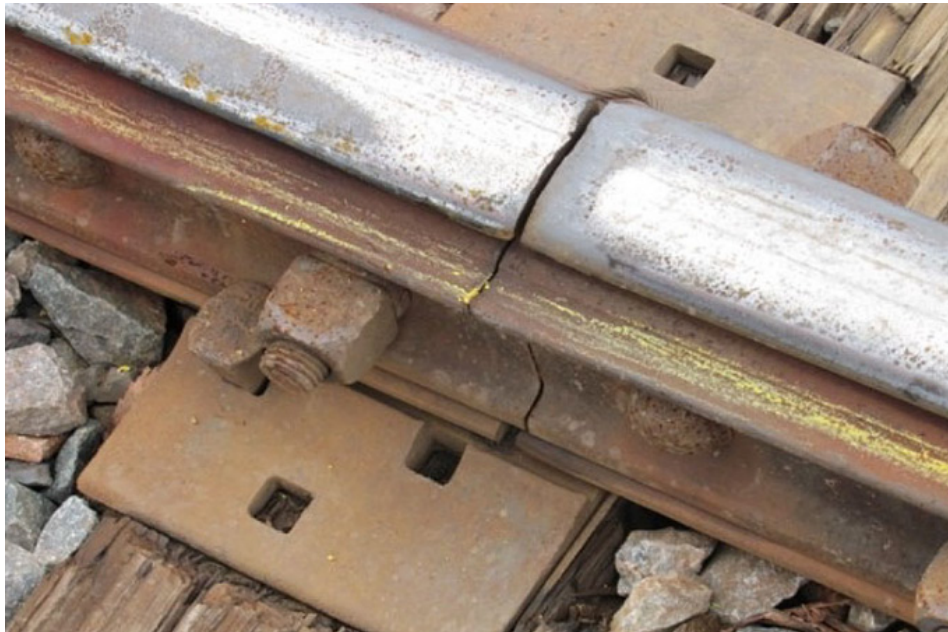
Figure 6.6.3-6 Track Asset Deficiency: Joint Defect
