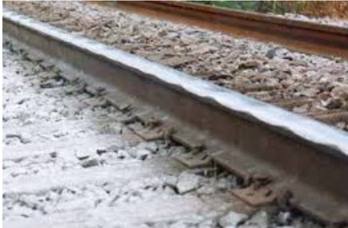
Figure 6.6.3-5 Track Asset Deficiency: Corrugation
