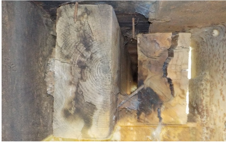
Figure 6.2.4-2 Timber Deficiency: Cracks and Splits
