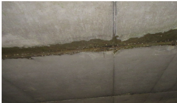
Figure 6.2.1-8 Concrete Deficiency: Differential Settlement
