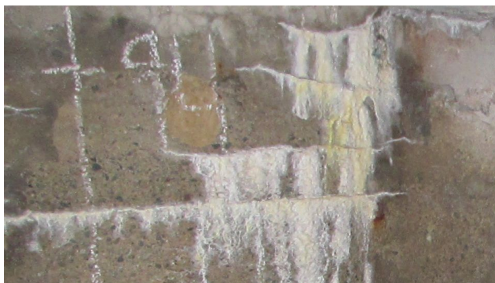
Figure 6.2.1-5 Concrete Deficiency: Efflorescence
