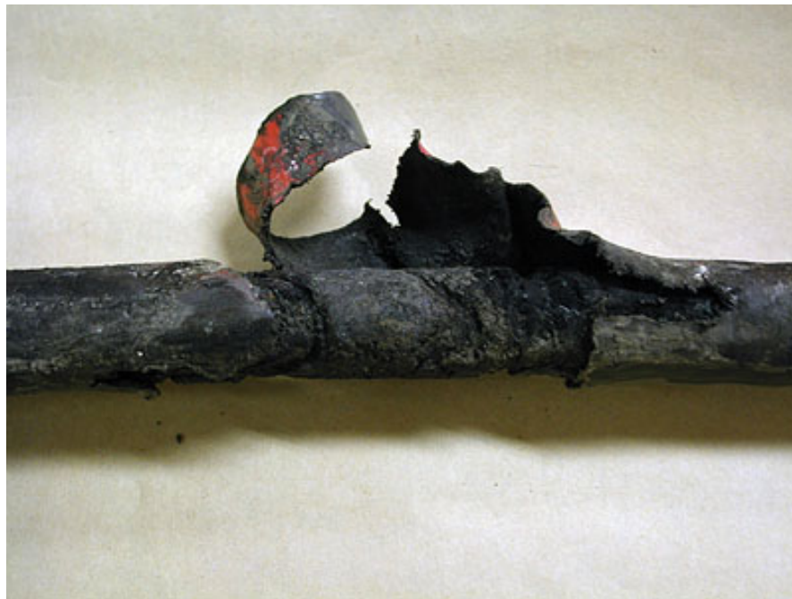
Figure 6.6.2-2 Power Asset Deficiency: Signs of Arcing on Cable
