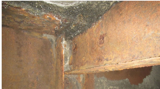
Figure 6.2.2-2 Steel Deficiency: Moderate Corrosion
