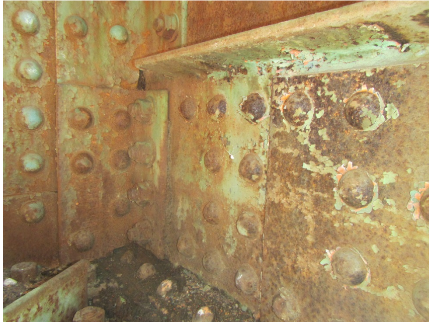
Figure 6.2.2-4 Steel Deficiency: Connection (Light Corrosion)
