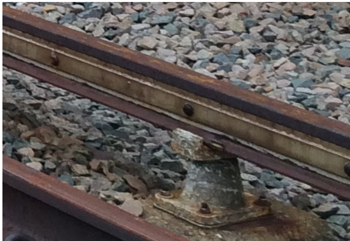
Figure 6.6.3-7 Track Asset Deficiency: Cable
