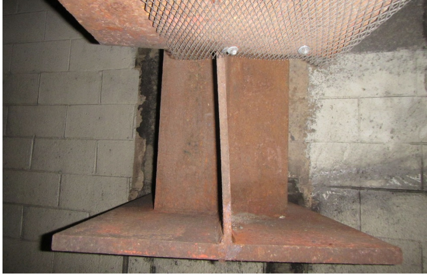
Figure 6.2.2-5 Steel Deficiency: Distortion
