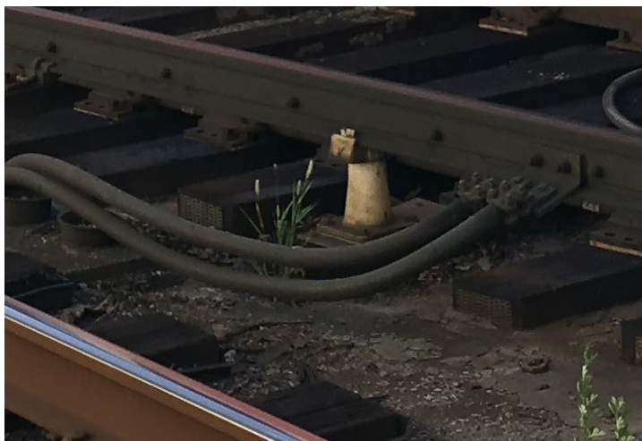
Figure 6.6.3-8 Track Asset Deficiency: Cable
