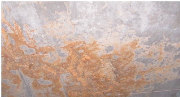
Figure 6.2.1-4 Concrete Deficiency: Rust Staining
