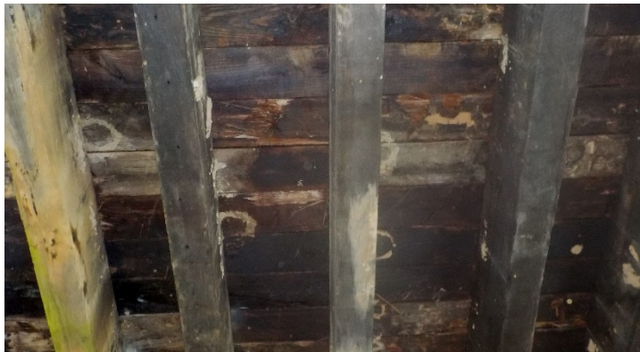
Figure 6.2.4-1 Timber Deficiency: Decay or Rot
