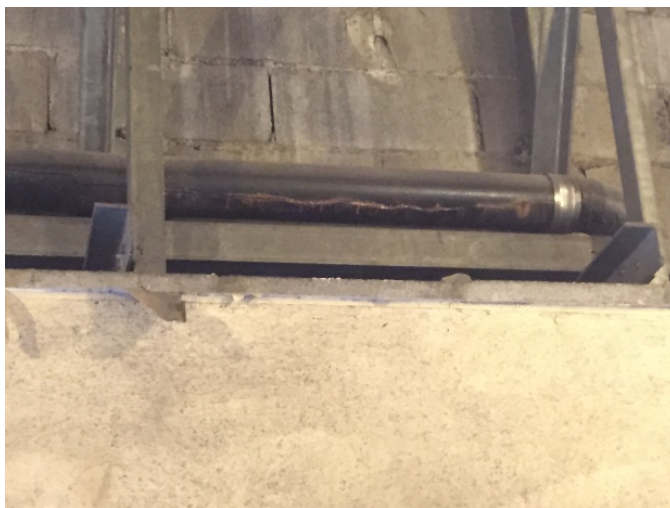
Figure 6.3.1-1 Drain System Deficiency: Cracked Pipe
