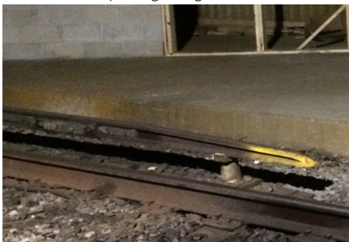
Figure 6.6.3-10 Track Asset Deficiency: Cable
