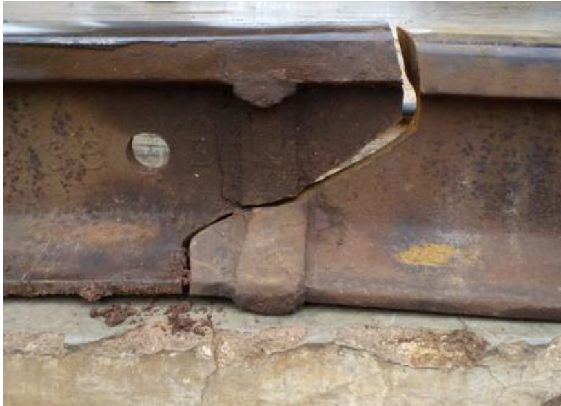
Figure 6.6.3-2 Track Asset Deficiency: Weld Failure
