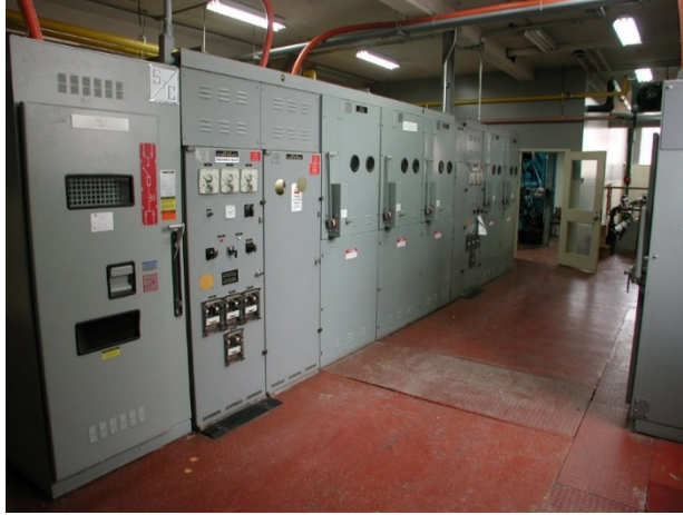
Figure 6.6.2-6 Typical Electrical Room
