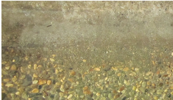
Figure 6.2.1-6 Concrete Deficiency: Scaling
