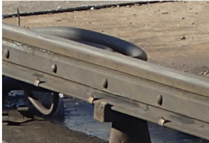
Figure 6.6.3-11 Track Asset Deficiency: Cable
