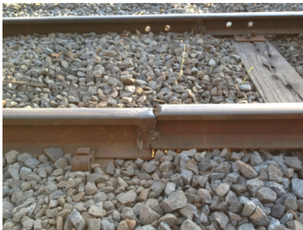
Figure 6.6.3-1 Track Asset Deficiency: Broken Rail
