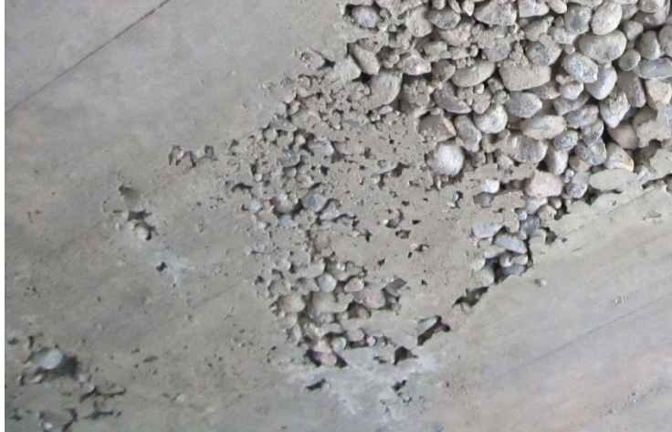
Figure 6.2.1-7 Concrete Deficiency: Honeycomb
