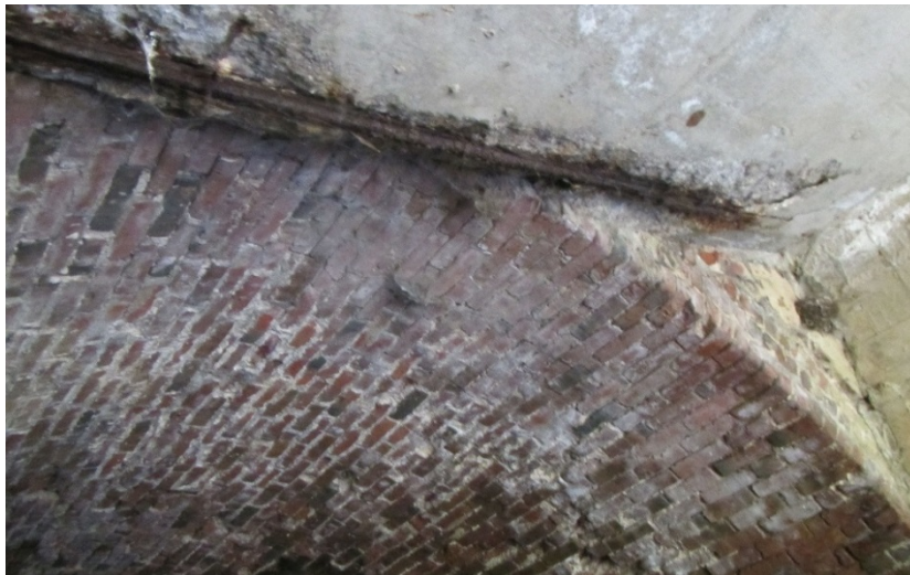
Figure 6.2.3-1 Masonry Deficiency: Mortar Breakdown and Efflorescence
