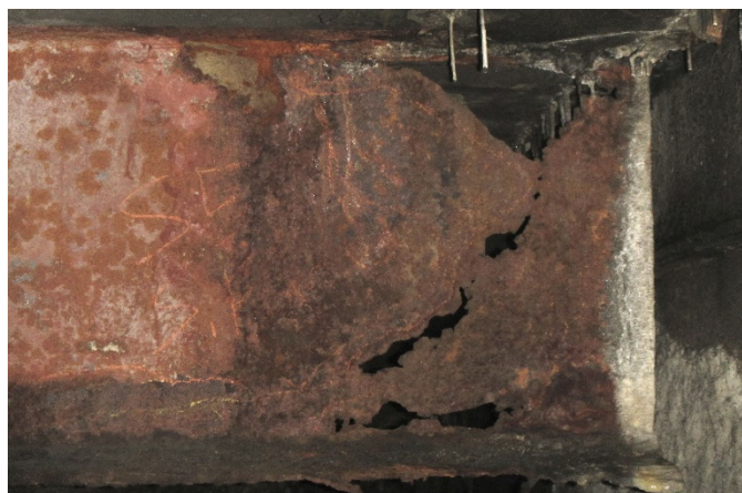
Figure 6.2.2-3 Steel Deficiency: Severe Corrosion
