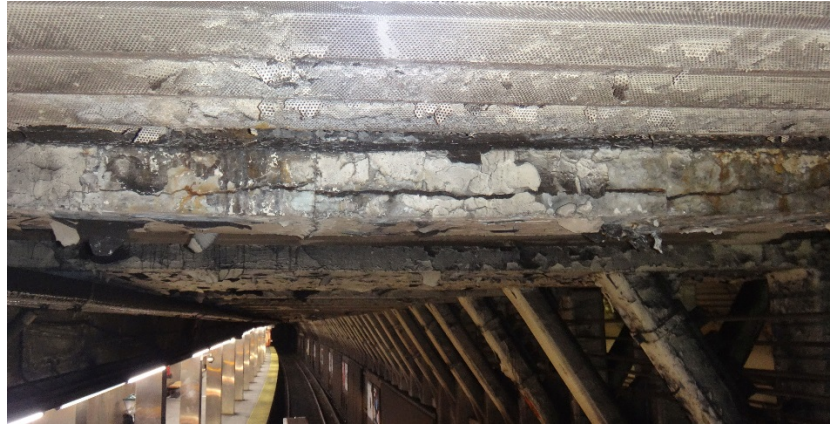
Figure 6.2.1-9 Concrete Deficiency: Incipient Spall at Concrete Encased Steel Beam
