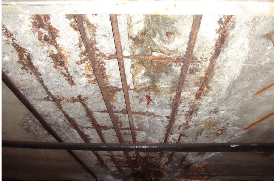
Figure 6.2.1-1 Concrete Deficiency: Spall with Exposed Reinforcing Steel
