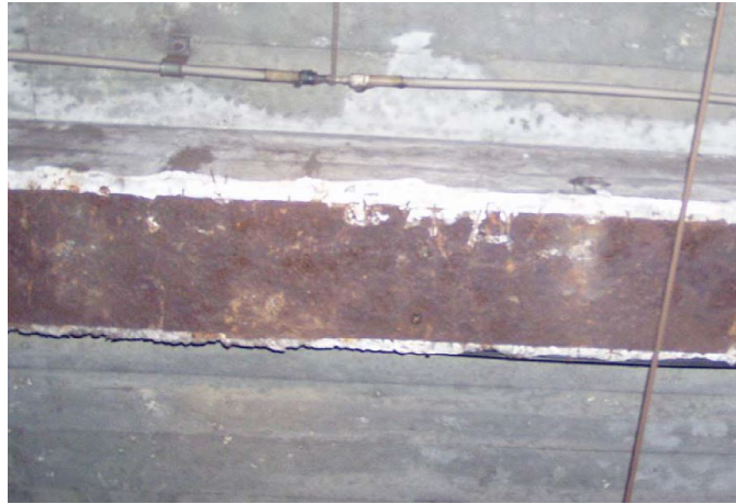
Figure 6.2.2-1 Steel Deficiency: Light Corrosion
