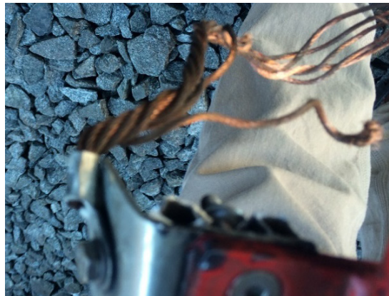
Figure 6.6.2-4 Power Asset Deficiency: Frayed Conductor
