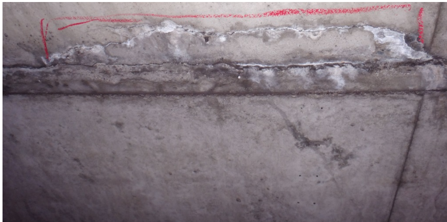
Figure 6.2.1-2 Concrete Deficiency: Delamination
