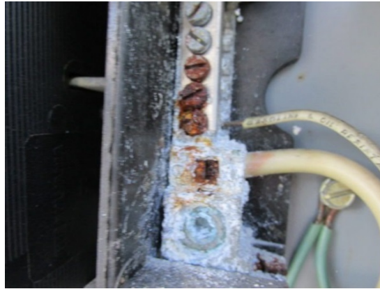
Figure 6.6.2-3 Power Asset Deficiency: Corrosion
